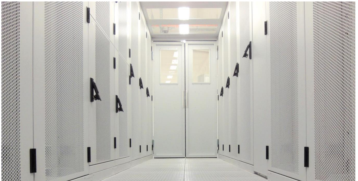
The above image shows the inside of an air-conditioned Swisscom server room in Zurich Herdern.
